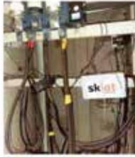
The device helps detect faults in electrical lines and power equipment in real time
