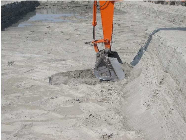
Fig 3.2(b) Collection of ash from the pond at Ramagundam
