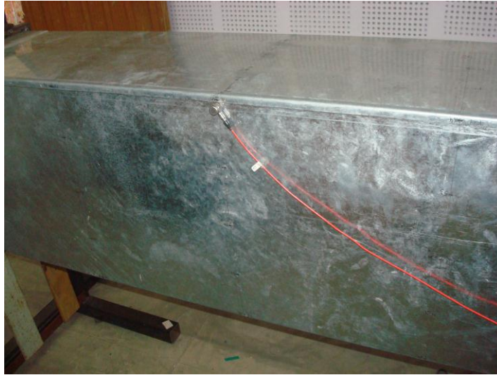
Figure 3.17b: Accelerometer mounted on the duct
