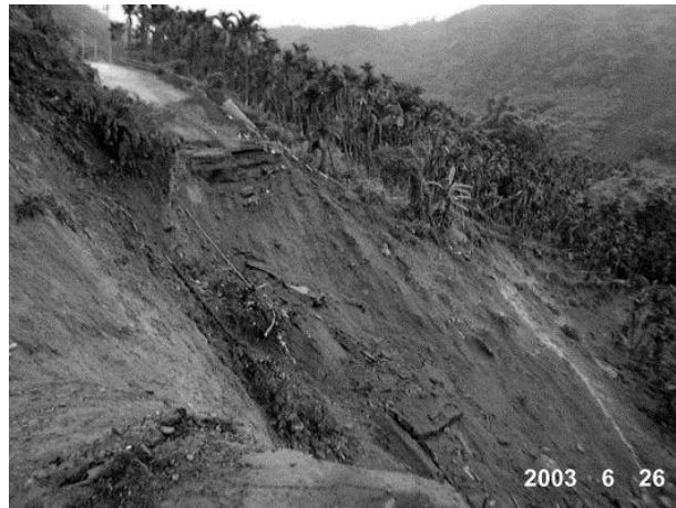
Figure 1.2: Failure of Earthen Embankment in Woo-wan-chai Area, Mt. Ali Road, Taiwan [2]
