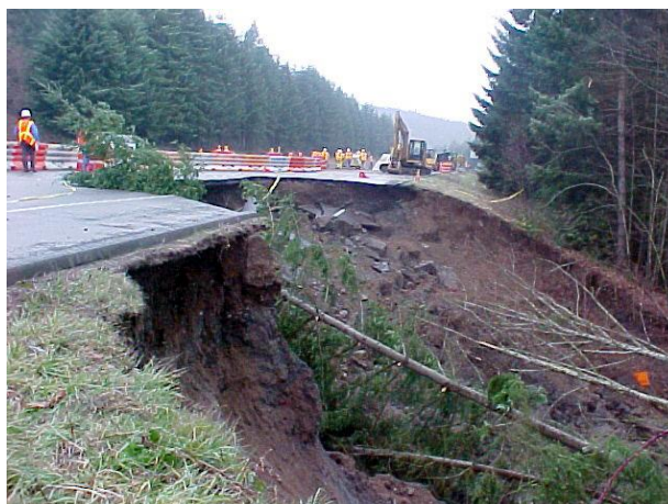
Figure 1.1: Failure of Highway 101 road embankment, Olympia, USA [1].
