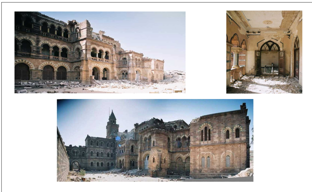
Figure 1.1: Photo of Prag Mahal (Bhuj, Gujarat, India) damaged in 2001 Gujarat Earthquake, Photo courtesy: Randolph Langenbach / UNESCO.
