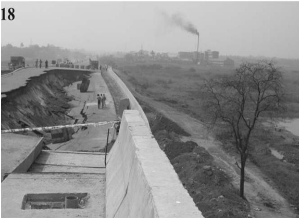
Figure 2.2: Failure of embankment right after construction
