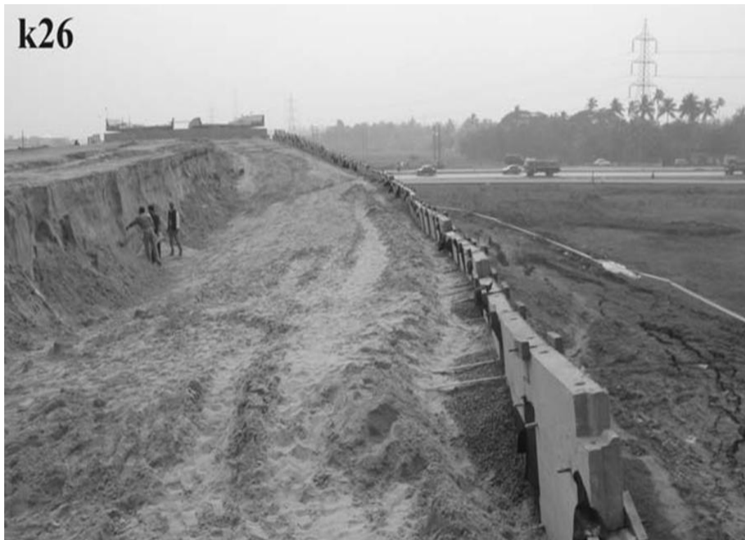
Figure 2.1: Failure during final stage of the embankment
