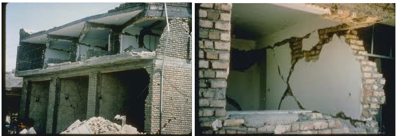
Figure 1.2 failures of the masonry walls due to earthquake [Geo hazard index html]
