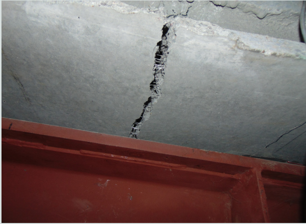
Tension side (crack arresting of fibers)
