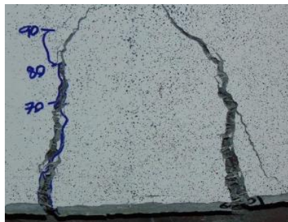
b) at major flexural crack location
