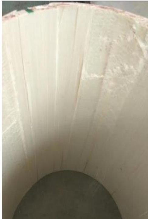
Figure 138 Presence of material imperfection and failure near stain gauge 4 and 5 (inside view)
