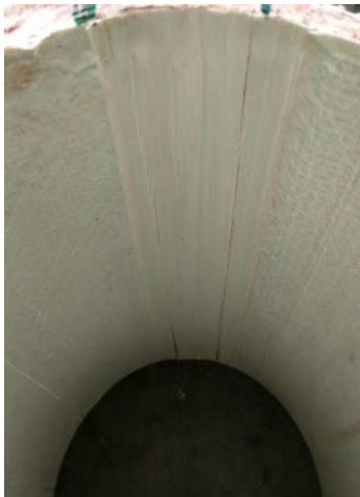
Figure 139 Presence of material imperfection and failure near stain gauge 1 and 2 (inside view)
