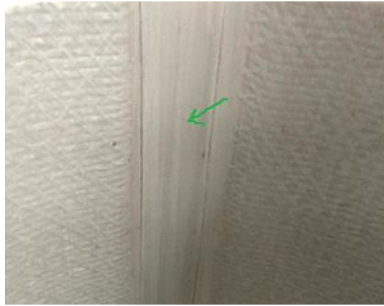
Figure 12 Presence of imperfection in pipe section
