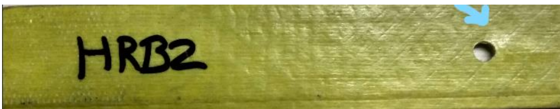
Figure 118 Bearing failure observed in HRB2
