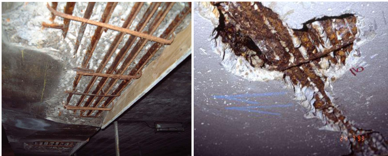
Figure 1. 1: Spalling of concrete due to corrosion ( www.ronacrete.co.uk )
