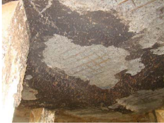
Figure 3: Spalling of cover concrete and exposure of rebar in the bottom of slab
