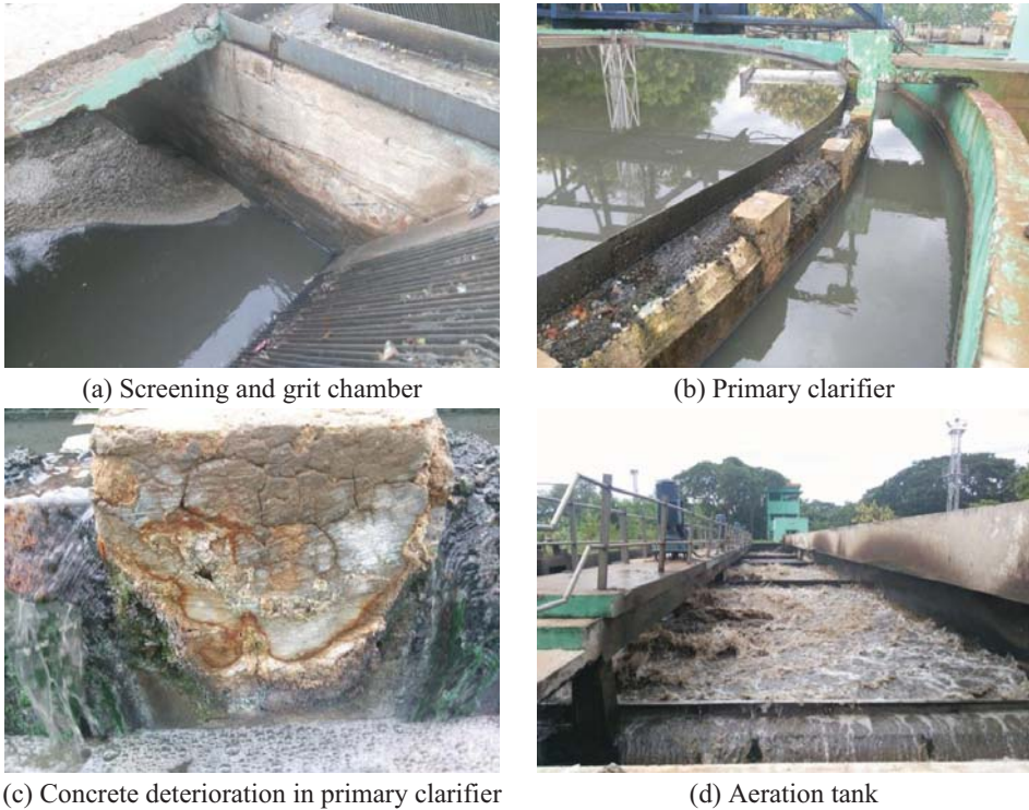
Fig. 2: Concrete deterioration in various locations of Nesapakkam sewage treatment plant
