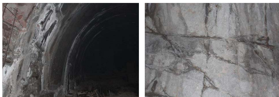
Figure 1: View of underground reinforced concrete structures with damages associated with several types of corrosion actions
