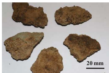
Fig. 2: Deteriorated concrete samples
