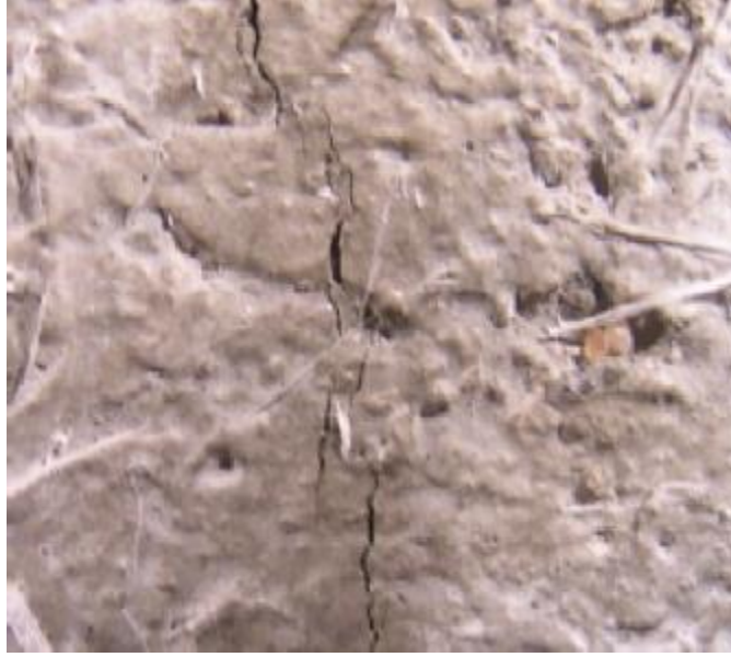
Figure 2.8: Plastic shrinkage crack in the steel–polypropylene hybrid concrete
