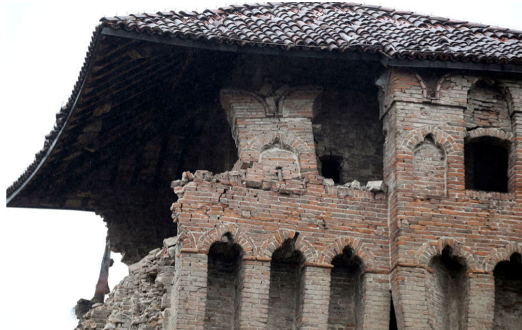
Figure 1.1: A earthquake-damaged Unreinforced Masonry building with an out of plane collapse in Italy Photo courtesyRoberto Serra/Iguana Press/Getty
