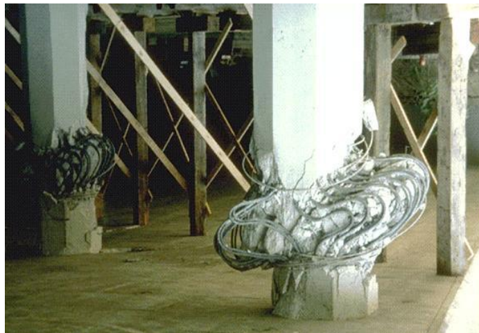
Figure 1.1 Plastic hinge in column (Source: earthquake.usgs.gov)
